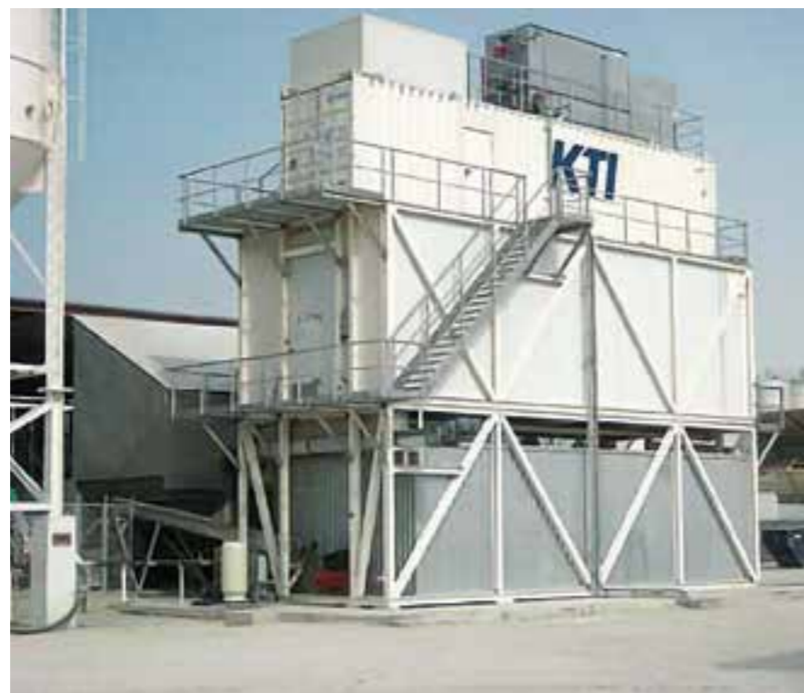
Combined Ice Water / Flake Ice Plant
