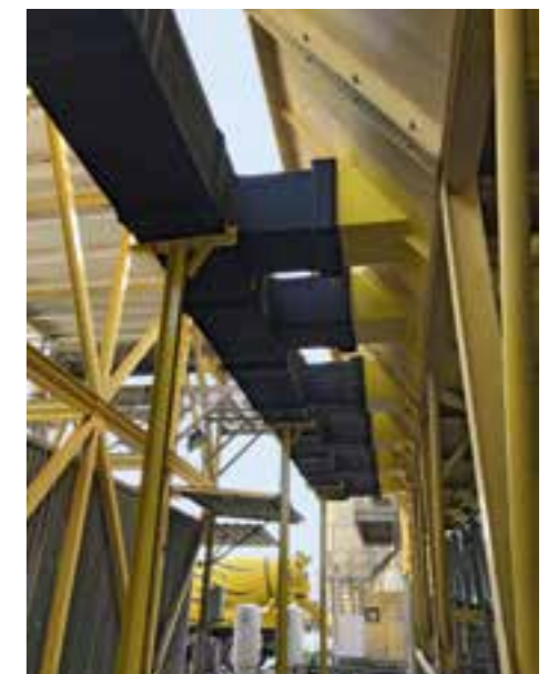
Live image of ductwork for cold air supply
