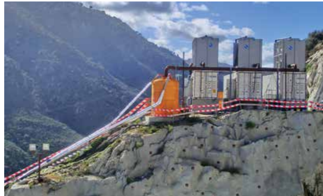
Cold water plants on the edge of a hydropower dam
