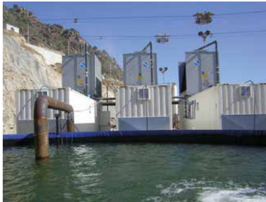
Cold water plants with re-circulation water basin for post-cooling
