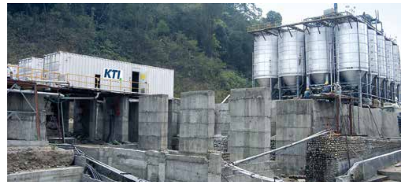
Flooded silo system with KTI water chillers for aggregate cooling
