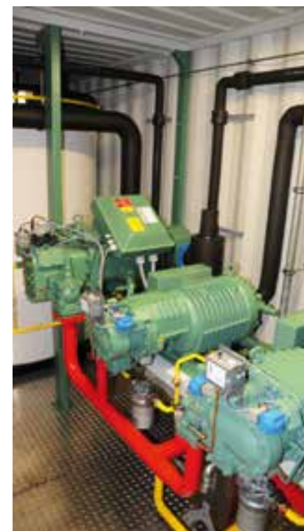
Flake ice maker with compressor units and oil separator
