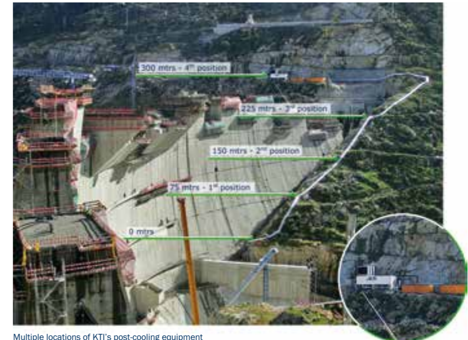
Multiple locations of KTI's post-cooling equipment
