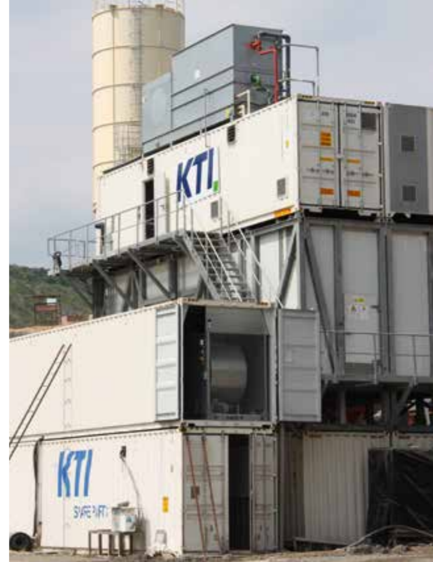
2x PLIP 100 on top of MIS 75 and Cold Water Plant beside
